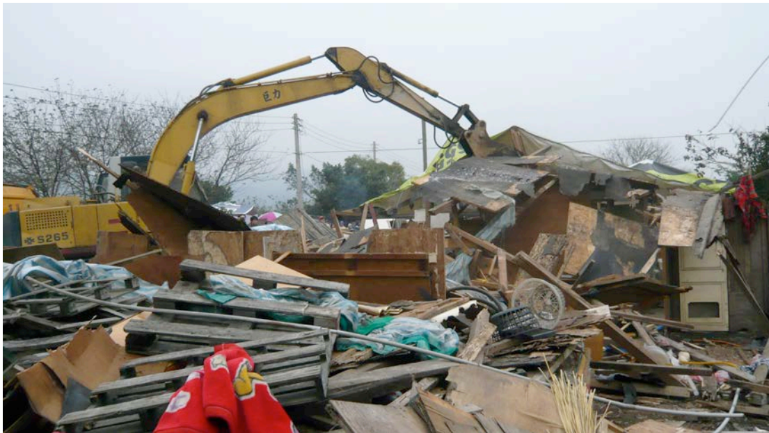
Fig. 5: Government bulldozers destroyed Fangas, the other Amis waterfront community, in 2008. Photo: Yu Xin-ke.
